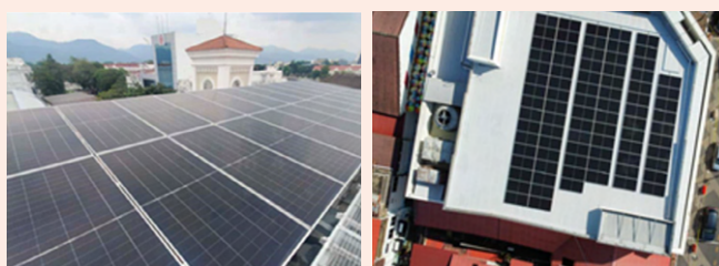
Solar panels installed at our OCBC Ipoh (left) and Muar (right) branches.
