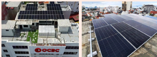
Solar panels installed at our OCBC Penang branch.
