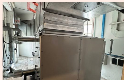
An upgraded AHU air-conditioning unit at Menara OCBC.
